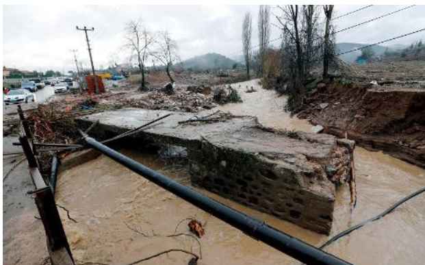
Figure 8: Flood damage in Menderes District, Izmir, Turkey, 02 February 2021. Photo credit: Izmir Governorship/Izmir Valiliği
