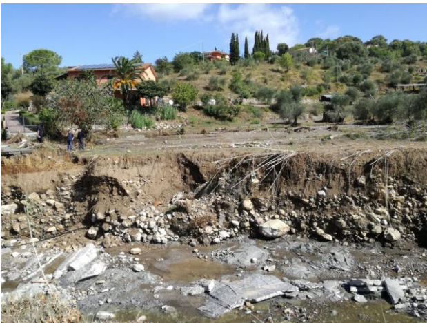
Figure 8. Floods destroyed a bridge over the Ardenza river. Taken on 12 September, 2017. Photo credit: Regione Toscana, Under Creative Commons CC BY-NC-ND 2.0
